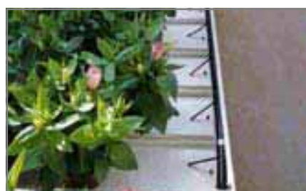
Gutter with running water
