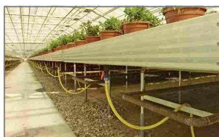
Heating for roller bench installations
